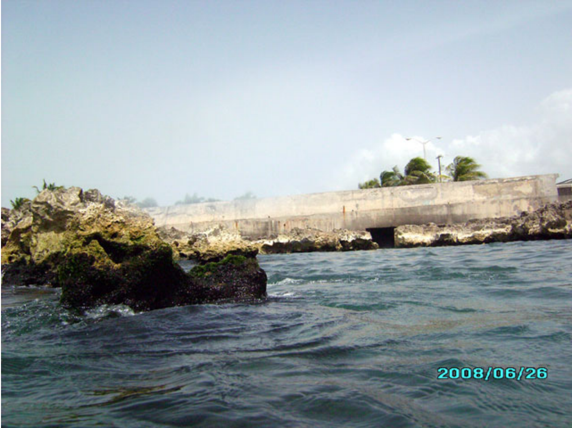
Directly in front of the outfall (square black hole in the wall) a rock reaches the surface
