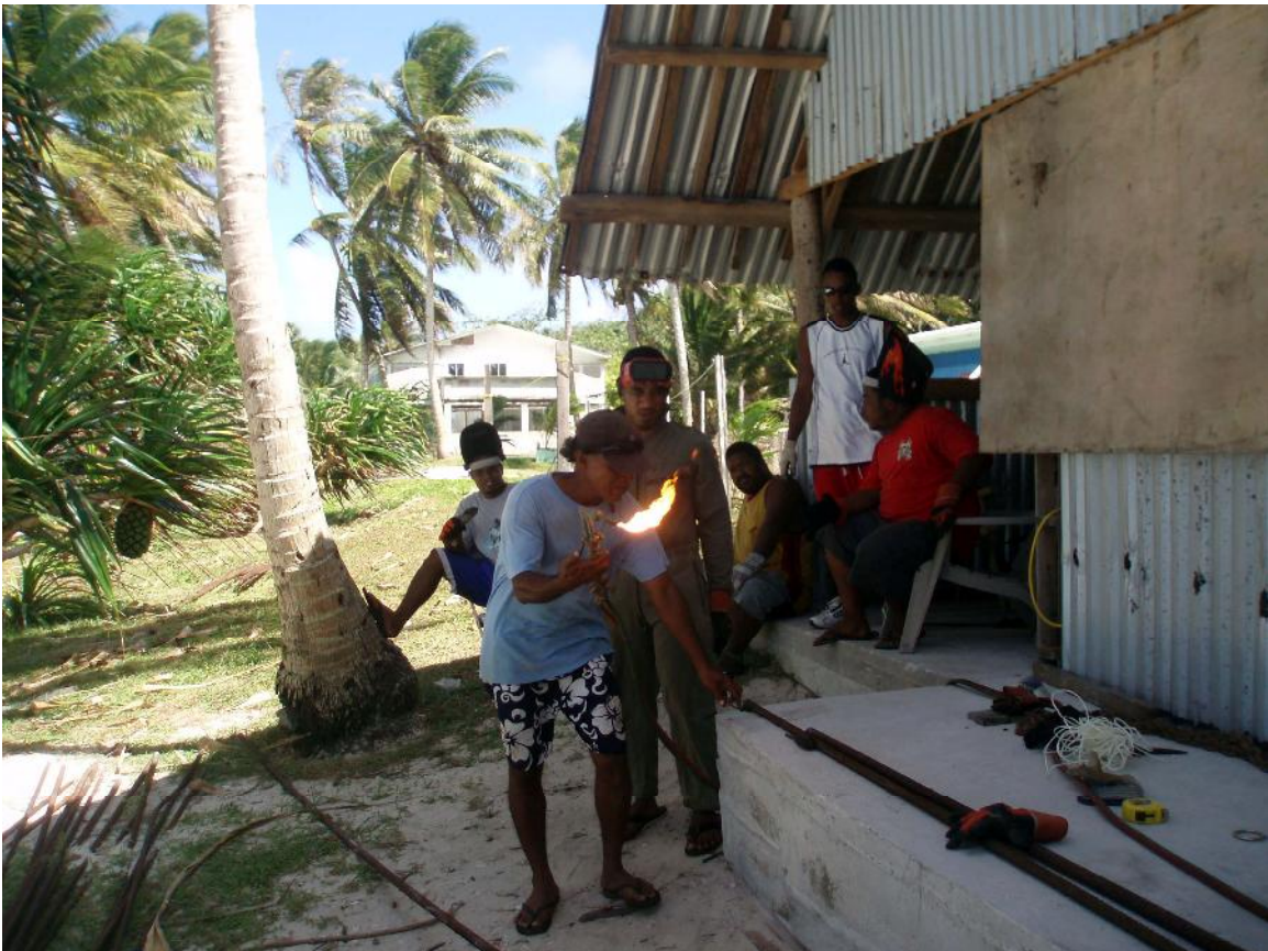
Figure 2. Workshop facility constructed at Jabo Village, Arno. Katwel Jormelu is shown training the local team in use of a gas torch to bend steel bars to make Biorock shore protection modules.
